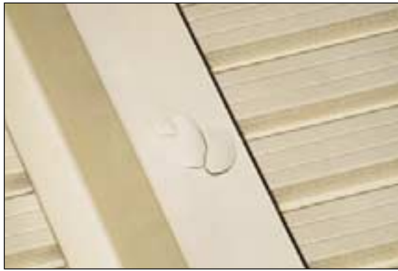
Fig. 4 - Steel exposed by thermal stress-induced blistering. (Note circular patterns relating to stepwise progression of failure.)
