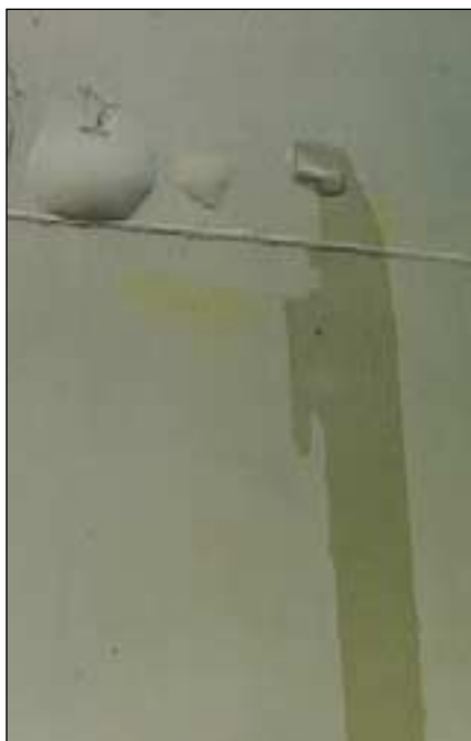
Fig. 3 - Blistering on tank exterior induced by thermal gradients. (Inside fluid was cold; outside environment was warm and humid.)
