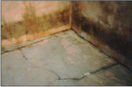
Cracks in the concrete flooring
