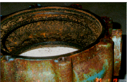
Corroded pump casing before preparation
