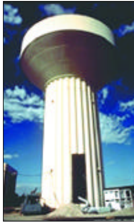
Water towers can be dehumidified through the bottom of the tower. Photos courtesy of Enviro-Air Corporation
